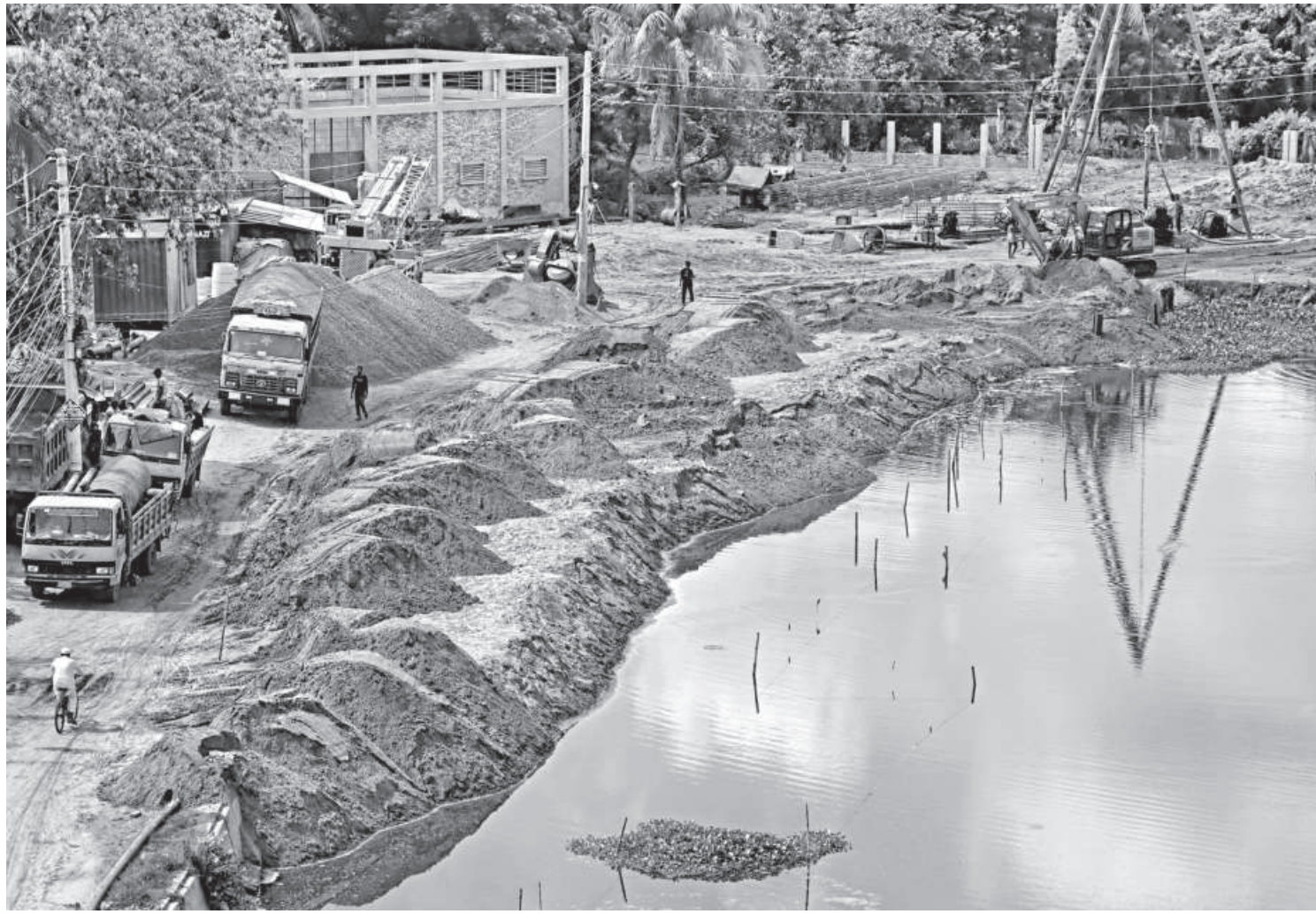
A part of the Nirala Dighi, the largest pond in Khulna city, is being filled up by the Khulna Development Authority for a road extension project.
