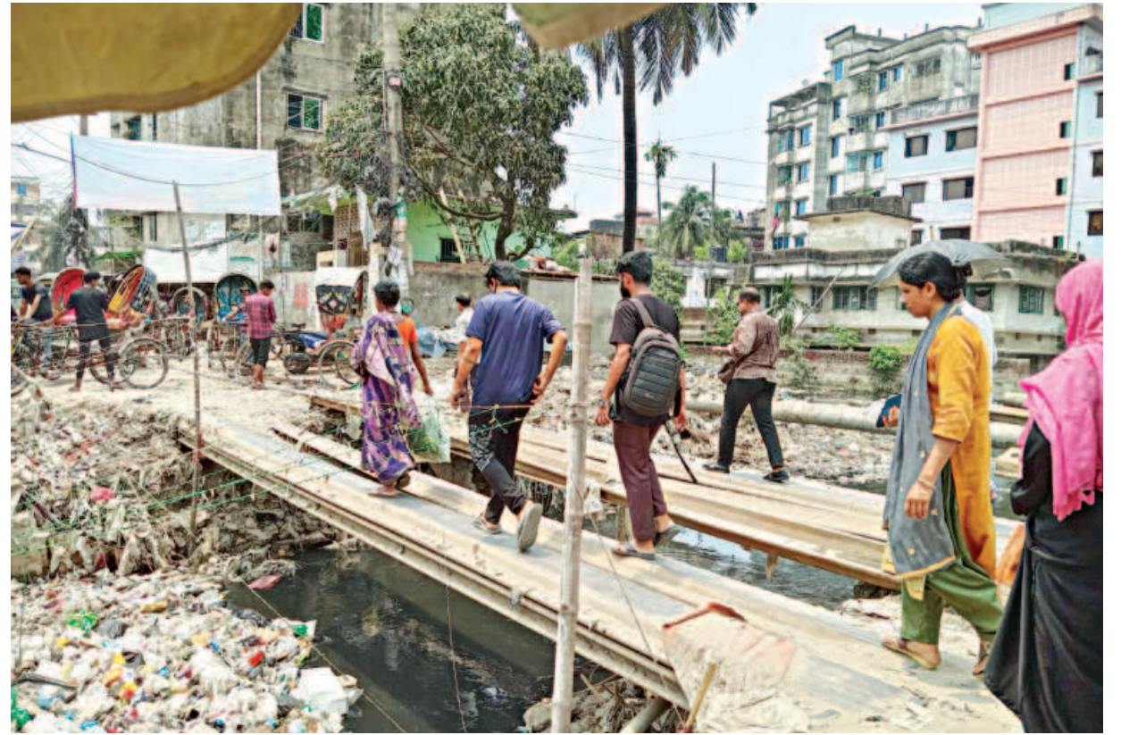
People cross this makeshift pathway, set up as part of ongoing works, in Chawkbazar Phooltala area. This temporary pathway not only makes it difficult for vehicles to cross, but also poses a risk to people as they can fall into the canal at anytime.
