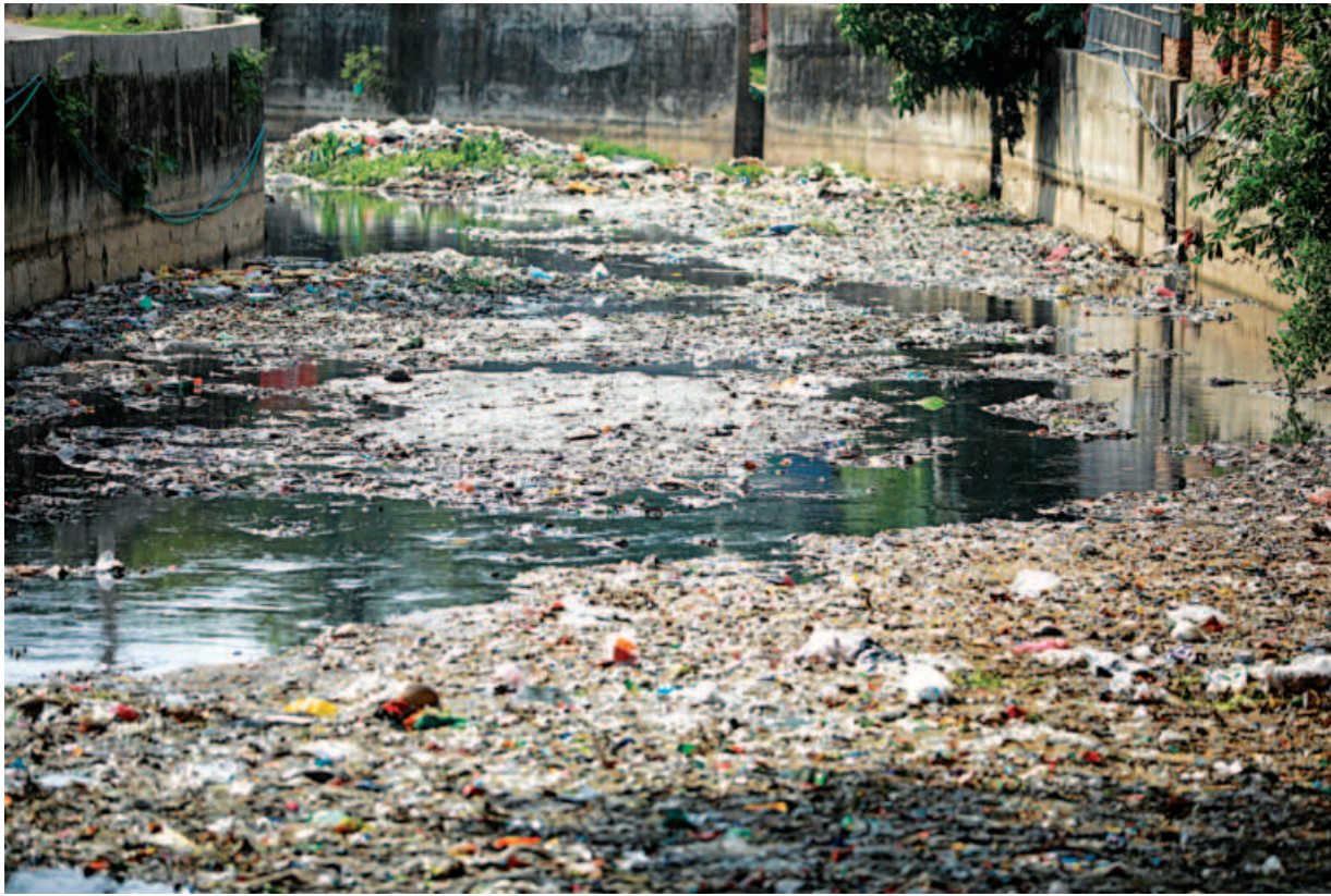
The loss of lives and civic hardships continue despite a Tk 8,626.62 crore mega project by the Chattogram Development Authority, which is currently underway, aimed solely at addressing waterlogging. This photo was taken recently in Ambagan Shaheed Lane area.
