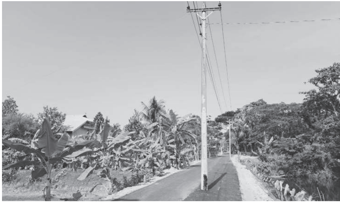
This electric pole is located on the middle of an approach road to a bridge on a canal in Char Montaj union of Patuakhali's Rangabali upazila. Despite construction work being completed six months back, the pole is yet to be removed.
