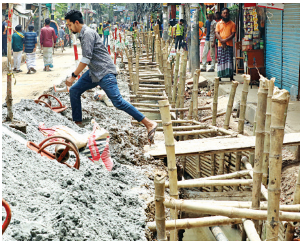
A man crosses a trench dug for installing underground power lines at Tikkapara in the capital's Mohammadpur. Locals said the work has been going on for around 25 days. The photo was taken yesterday.
