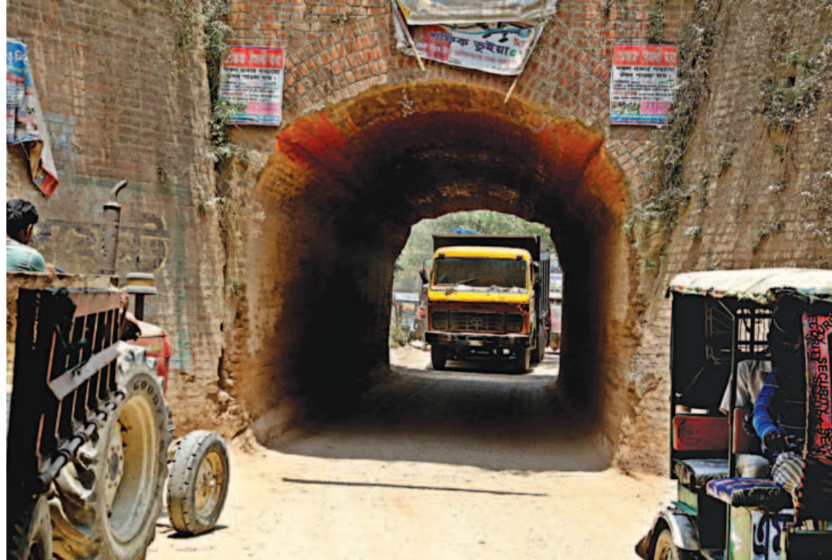
This small tunnel, built in the British era under a rail line, is key for various businesses in Ashuganj of Brahmanbaria to ship in and ship out goods. The old tunnel is getting damaged every day as heavy and tall trucks use the tunnel and scrape its ceiling. The photo was taken recently.
