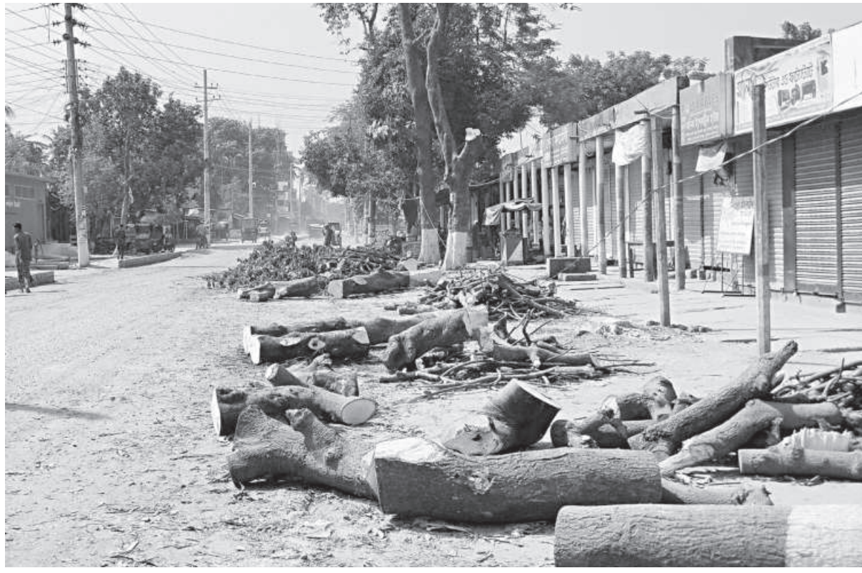
Not so long ago, many decades-old trees used to stand proud along the roadside and provide shade to commuters. However, at least 298 such trees are being felled for road expansion work at Bochaganj upazila in Dinajpur. Around 150 have already been already axed, according to locals. PHOTO: STAR
