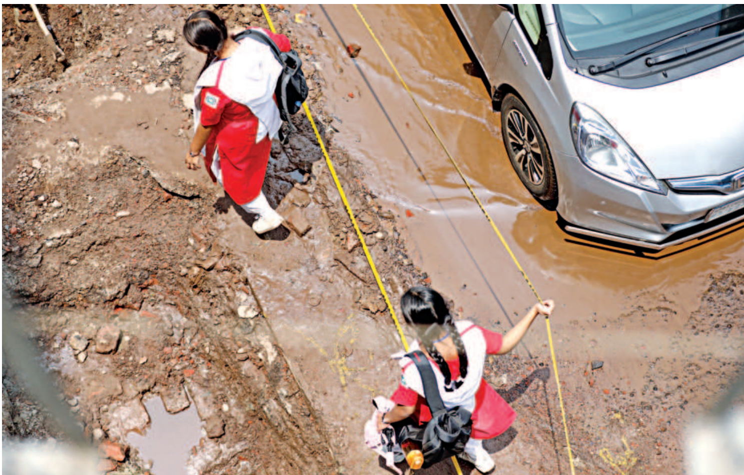
Two schoolgirls carefully walk on Motijheel-Tikatuli road, where DPDC is working on an underground power cable project for around a month. As a result, people are having difficulties commuting across the narrow road due to it being cut and frequent traffic jams. Besides, there are not much safety measures other than a flimsy yellow tape separating the project, posing risks to pedestrians and vehicles. The photos were taken yesterday.
