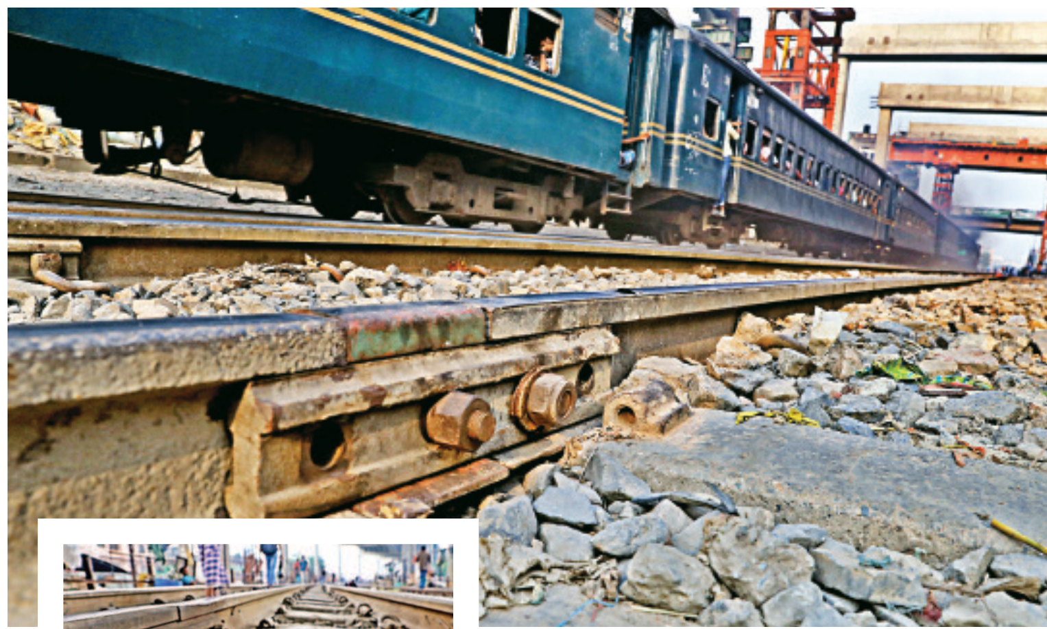
A fishplate, an irreplaceable component in railway tracks, with missing bolts near Malibagh rail crossing yesterday. Meanwhile, multiple clips, another vital part, have been absent from the tracks in Tejgaon railgate area, inset. This photojournalist noticed multiple such bolts and clips missing between the two spots. Such negligence can result in a mishap at any moment.
