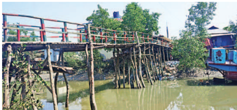
People of Chhota Baishdia union in Patuakhali's Rangabali upazila still use this ramshackle bridge on Gahinkhali Canal as authorities are yet to construct a new bridge, 12 years into declaring it abandoned. PHOTO: STAR
