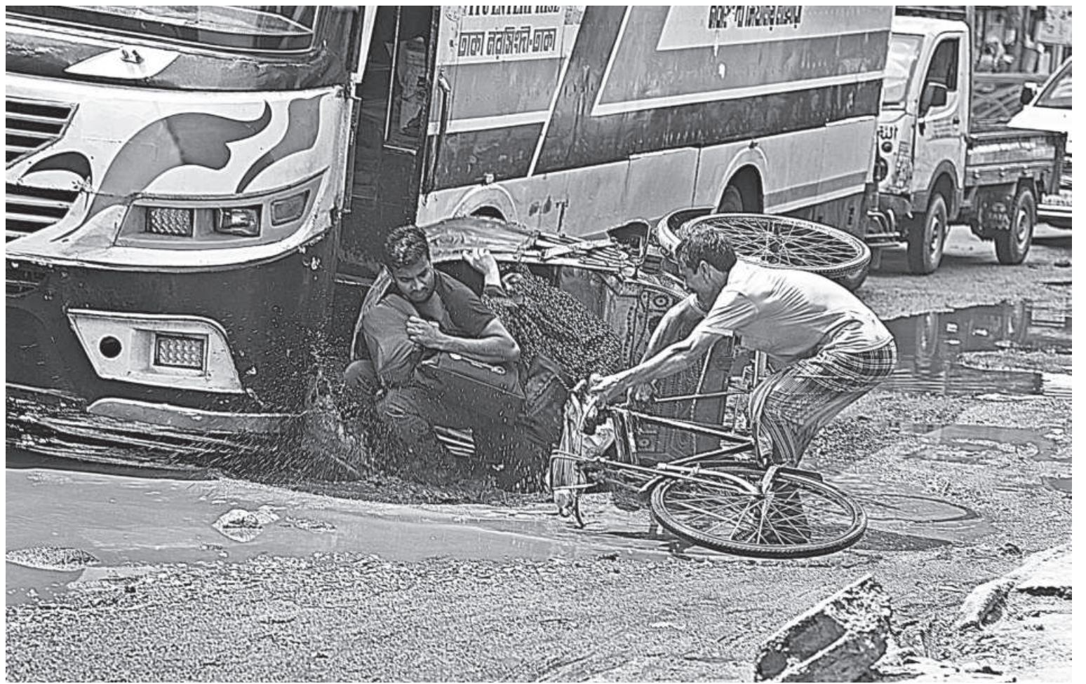
A rickshaw tips over as its wheel strikes a large pothole, while the passengers fall dangerously close to a moving bus on Hatkhola Road near the Tikatuli footbridge in the capital. The road was dug up for the installation of waterpipes and power lines about a month ago and has been in a dismal state since then, resulting in such accidents frequently. The photo was taken yesterday.
