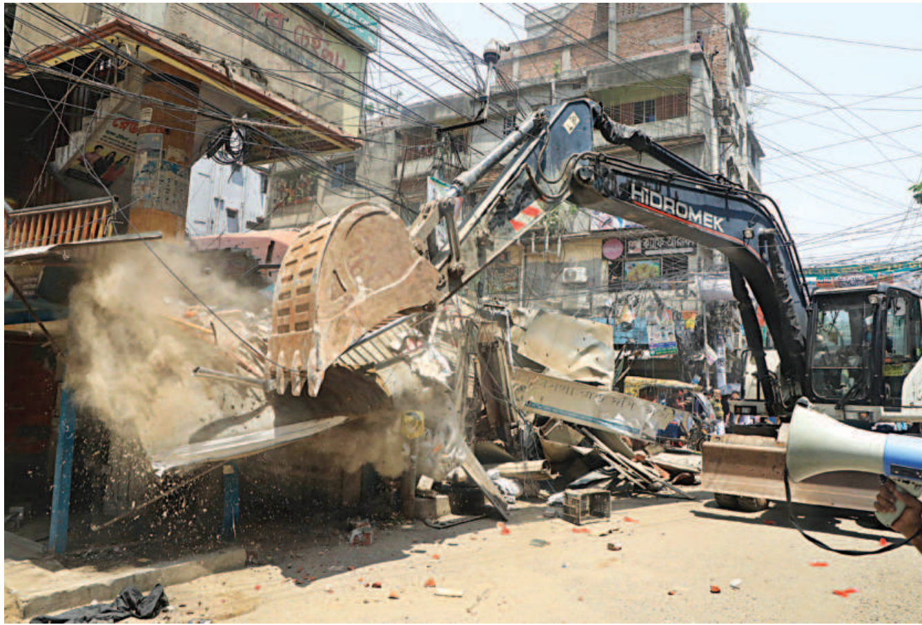
Dhaka South City Corporation starts demolishing illegal structures on both sides of Culvert Road in Uttar Mugdapara yesterday. Before the drive, the occupants of the structures were asked to move their belongings elsewhere.
