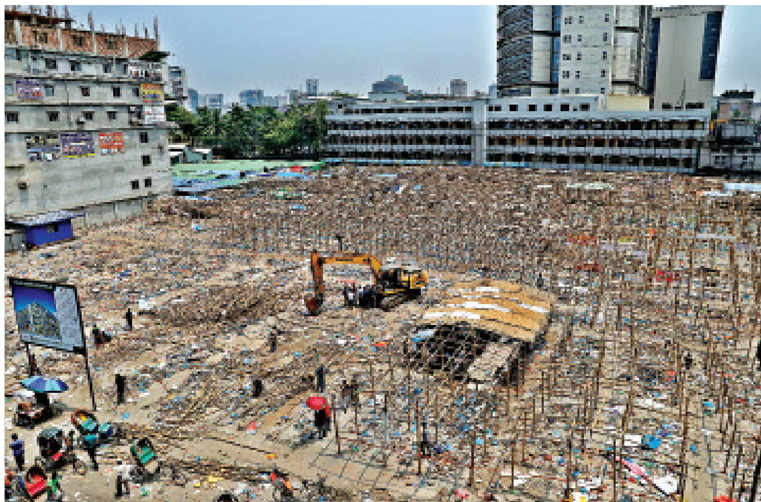
The DSCC continued the dismantling of the makeshift shops at the Bangabazar Shopping Complex for the second consecutive day yesterday. The shops were set up after a fire razed the market in April last year. Dhaka South Mayor Sheikh Fazle Noor Taposh had earlier announced that the construction work of Bangabazar market would start after Eid.
