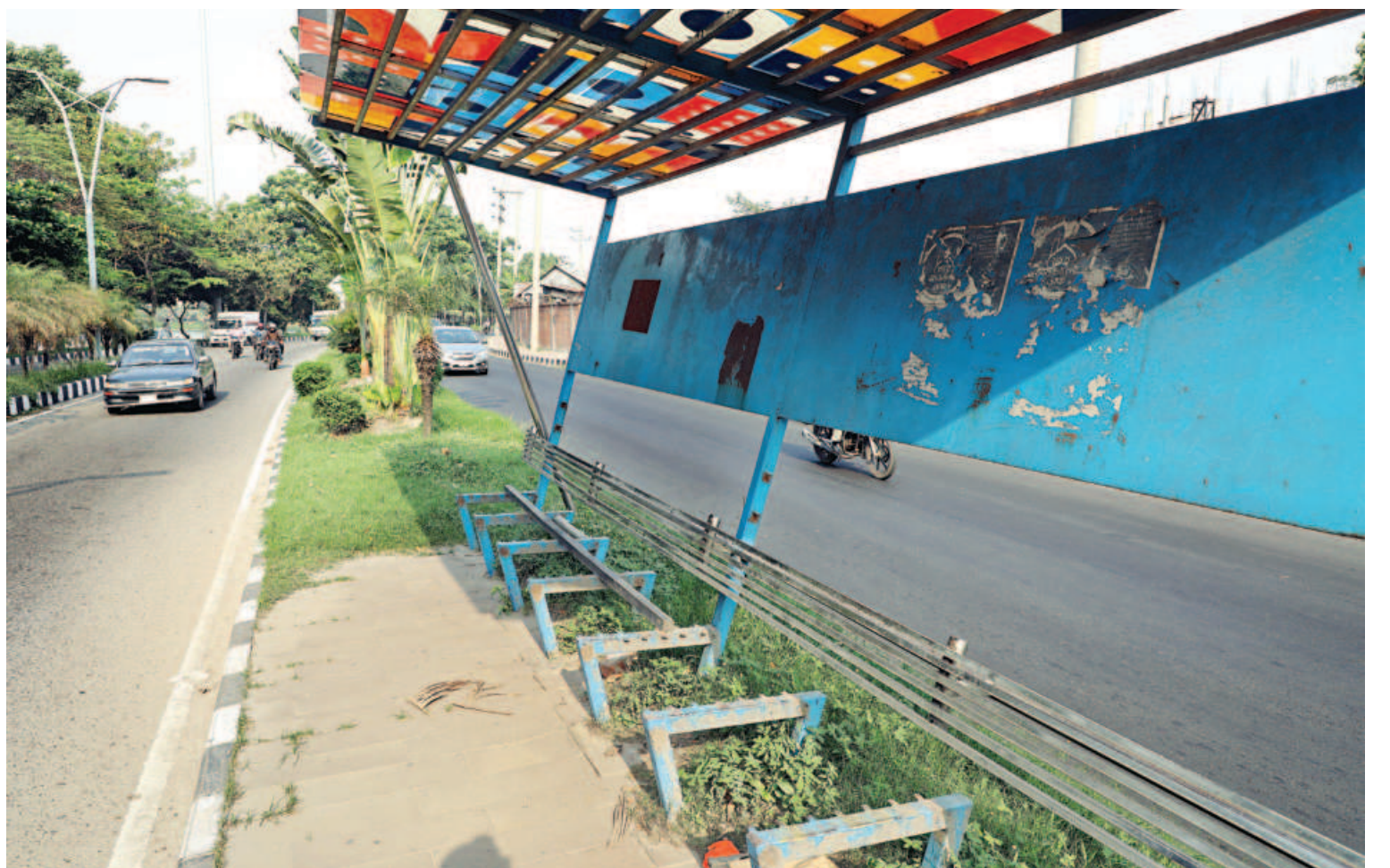
The seats of a bench at a bus stop in the capital's Hatirjheel seems to have disappeared amid a lack of monitoring and maintenance, making it unfit for use. However, any initiative to renovate the structure is yet to be taken, compelling passengers to stand for long hours while waiting for the bus. The photo was taken in Modhubagh area yesterday.
