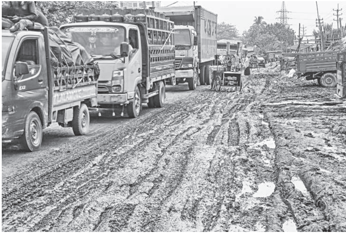
A long tailback on Sadar Ghat-Gabtol-Beribadh road while a dilapidated unusable part of it remains vacant. The authorities turn a blind eye to this issue. The photo was taken from Rayer Bazar recently. PHOTO: RASHED SHUMON
