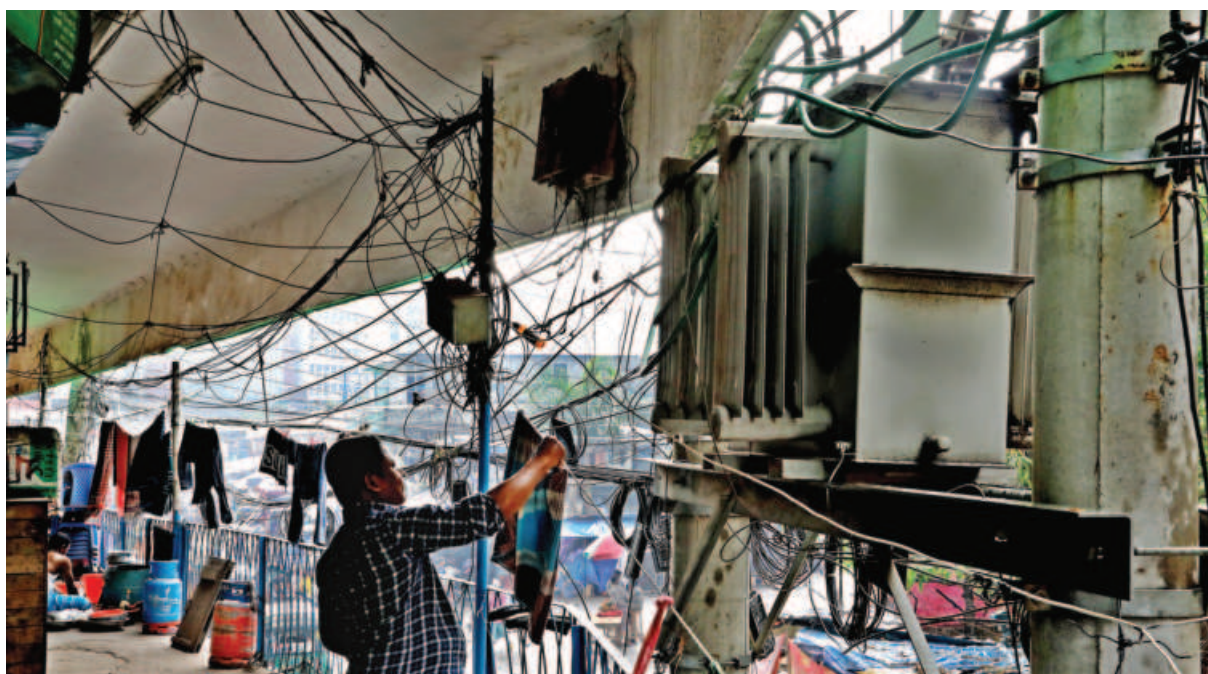
RECIPE FOR DISASTER ... A man hangs his wet clothes right next to an active electric transformer at the DIT Market in the capital's Karwan Bazar yesterday. In case of a transformer malfunction or spark, the clothes could catch fire, which could spread to the gas cylinders nearby and unleash a blaze.
