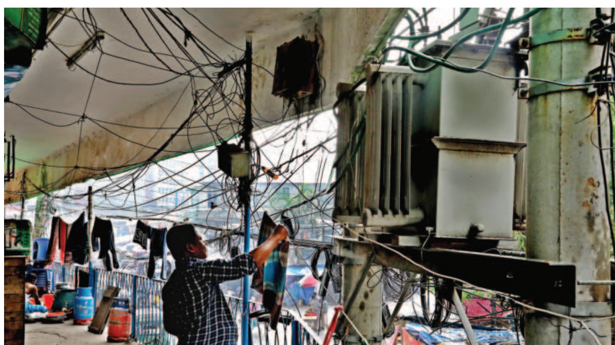
RECIPE FOR DISASTER ... A man hangs his wet clothes right next to an active electric transformer at the DIT Market in the capital's Karwan Bazar yesterday. In case of a transformer malfunction or spark, the clothes could catch fire, which could spread to the gas cylinders nearby and unleash a blaze.
