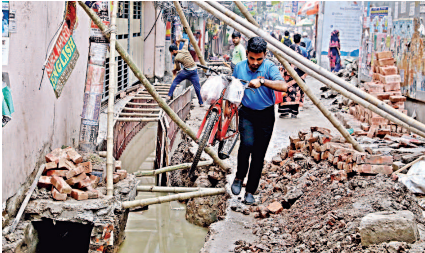
The Siddehswari Lane in Dhaka has been dug for the construction of a drain by Dhaka South City Corporation, leaving the road almost impassable. Local residents, particularly children and the elderly, are enduring suffering due to such unplanned development work.
