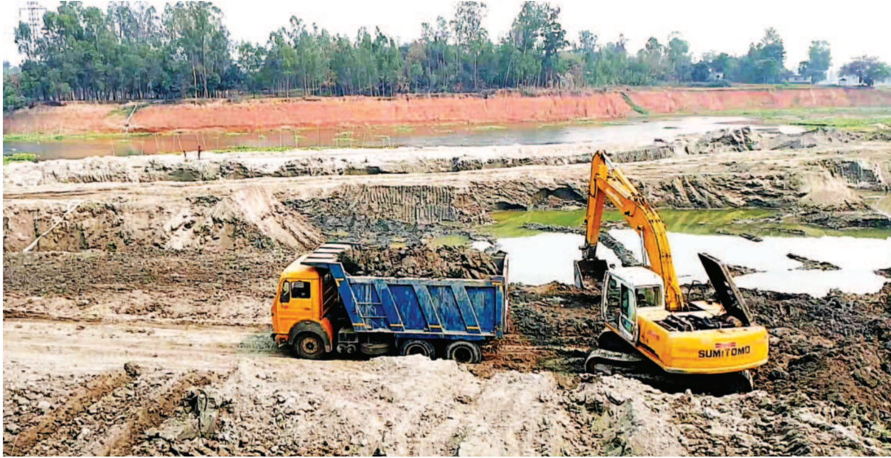
INVITING DANGER... Local influential people are illegally digging the bank of the Bangshi river at Chanpur in Tangail's Mirzapur upazila to collect soil and sell it for filling up low land, putting the entire area at risk of erosion. Collecting soil from river banks is prohibited under the Sand Quarry and Soil Management Act-2010. The photo was taken recently.
