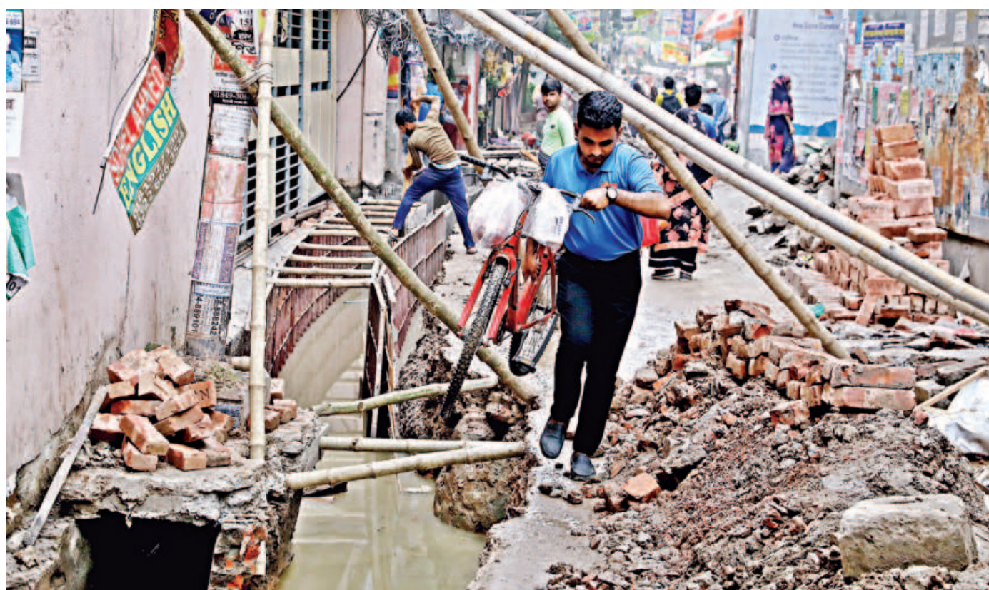
The Siddeshwari Lane in Dhaka has been dug for the construction of a drain by Dhaka South City Corporation, leaving the road almost impassable. Local residents, particularly children and the elderly, are enduring suffering due to such unplanned development work.
