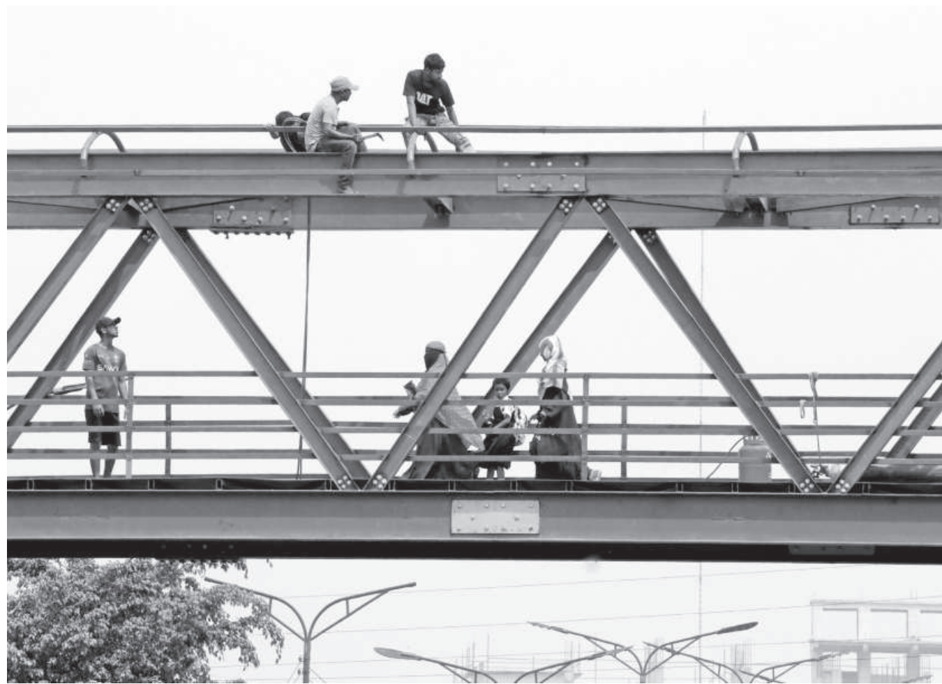
Workers welding the ceiling of a footbridge on Savar-Aricha highway while pedestrians, including children, pass from beneath. Their lack of safety gear and measures not just puts their life at risk but also compromises the safety of others. The photo was taken in Bank Town area, Savar yesterday.
