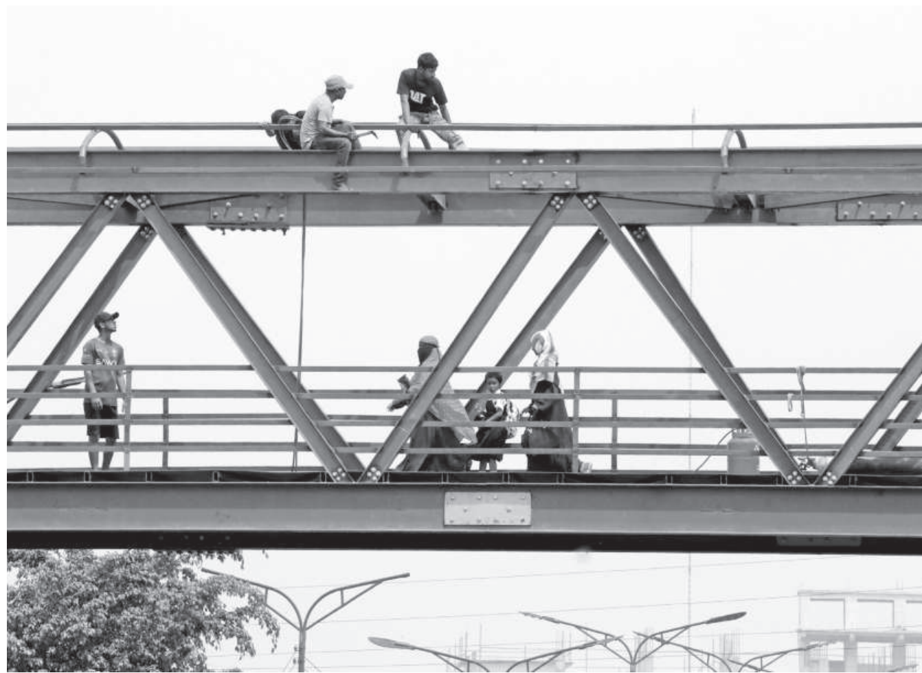
Workers welding the ceiling of a footbridge on Savar-Aricha highway while pedestrians, including children, pass from beneath. Their lack of safety gear and measures not just puts their life at risk but also compromises the safety of others. The photo was taken in Bank Town area, Savar yesterday.
