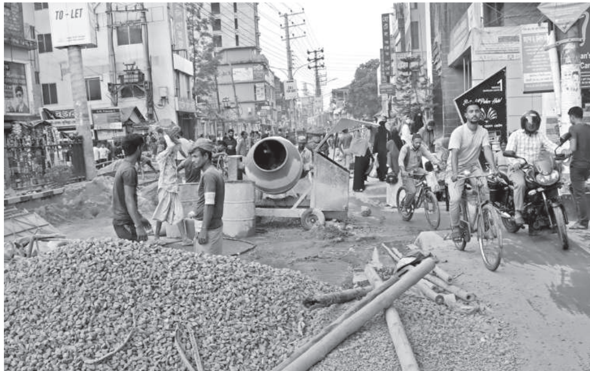
Pedestrians, motor bikers and cyclists take to the footpath as the Ambarkhana-Chouhatta road in Sylhet city remains blocked for road works, obstructing movement for all. Meanwhile, locals continue to use the road amid risks due to the absence of an alternative route. The photo was taken yesterday. PHOTO: SHEIKH NASIR
