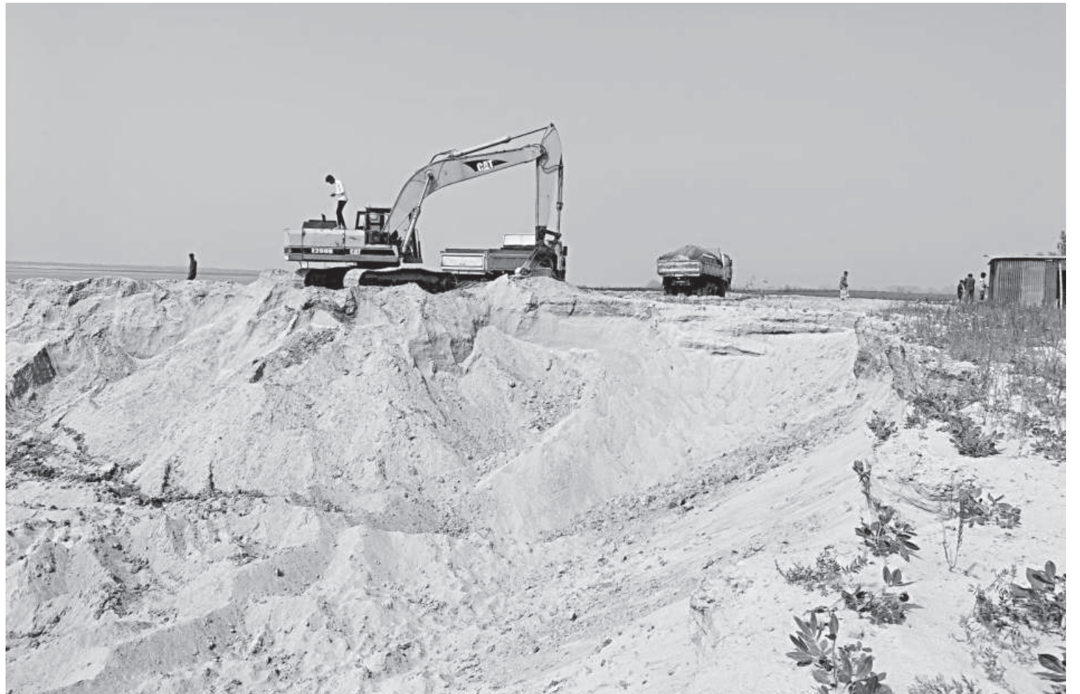
Excavators being used to extract sand indiscriminately from at least 10 points on the shoals of Jamuna river in Arjuna union of Tangail's Bhuanpur upazila.
