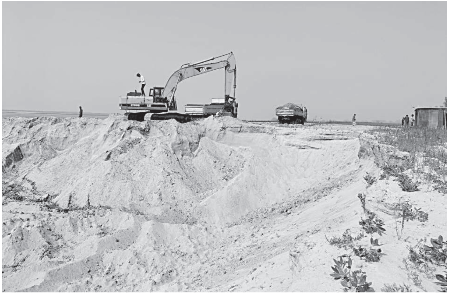
Sand being extracted illegally using an excavator on the shoals of Jamuna in Arjuna union of Tangail's Bhuanpur upazila. Locals say a group of influential people is lifting sand at nine more points in the area. PHOTO: STAR
