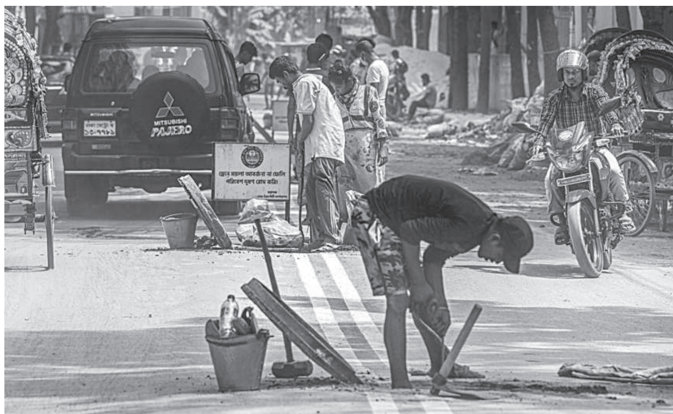
Workers cleaning sewerage lines as vehicles pass by on avenue-2 in Chondrima Model Town area of the capital's Mohammadpur yesterday afternoon. Their lack of safety gear and absence of demarcation around the open manholes further exacerbates risk of accidents.
