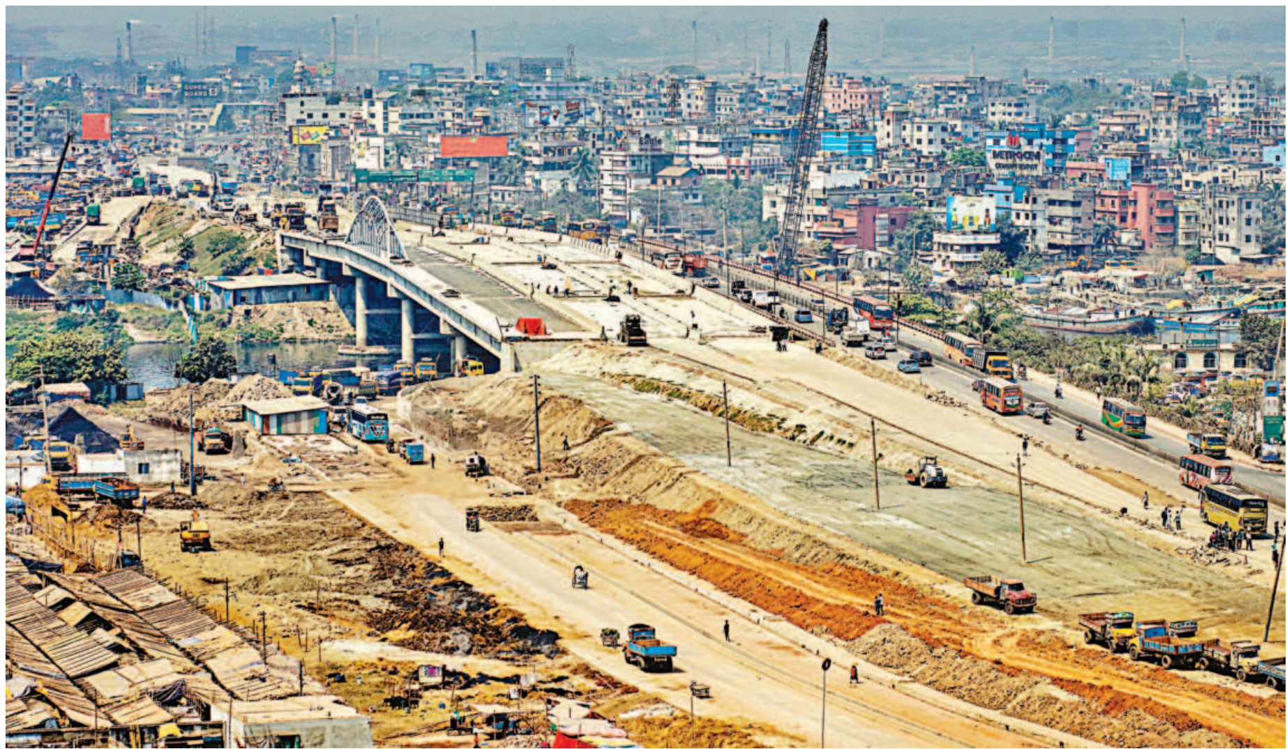
Construction of an eight-lane bridge along the existing one over the Turag near Dhaka's Aminbazar is underway. The Roads and Highways Department has sped up the work to open at least two lanes of the bridge on the Dhaka-Aricha highway before the Eid holidays. The photo was taken on Wednesday.
