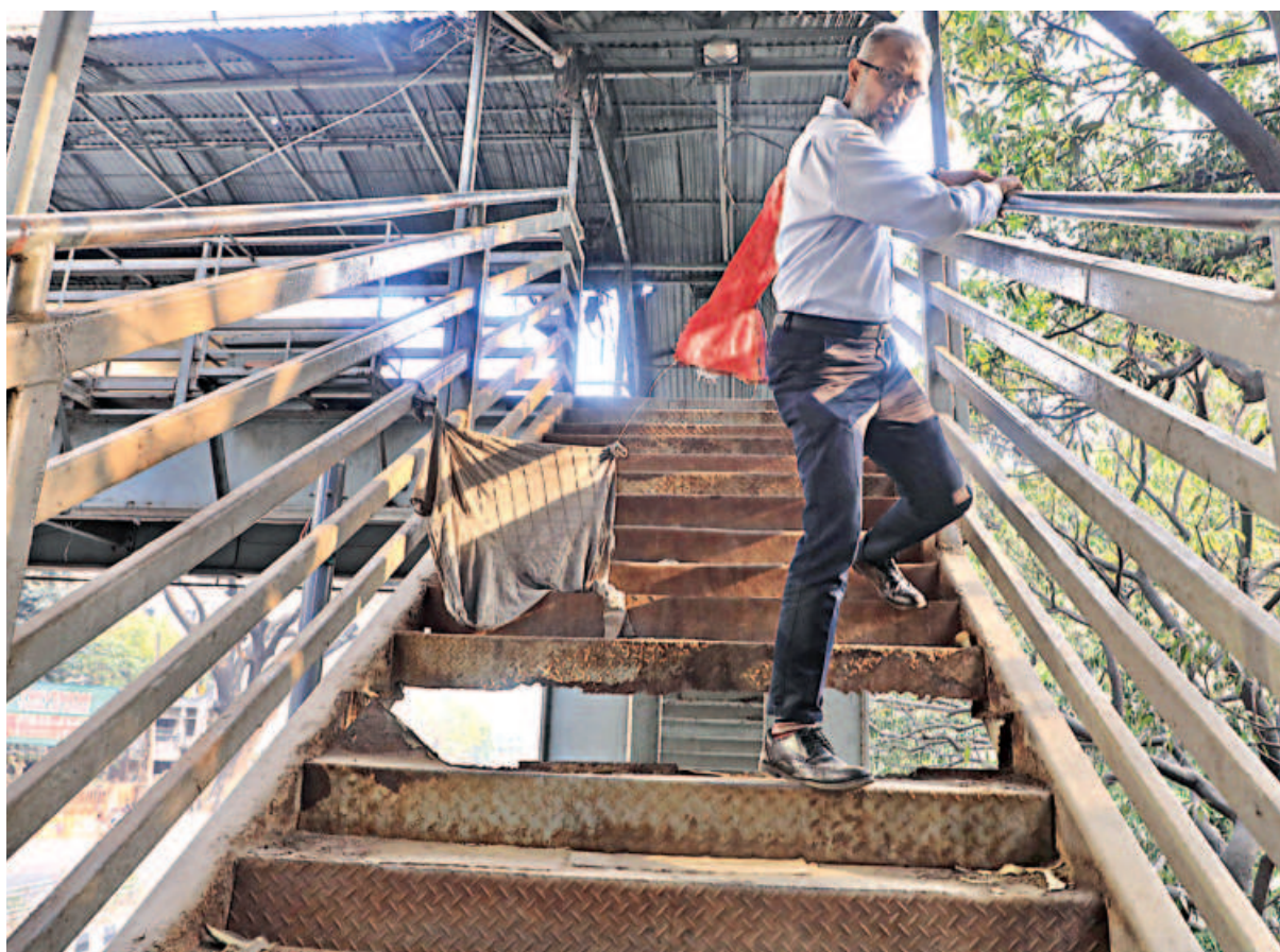
A pedestrian holds on strongly to the railing of the footbridge's staircase in the capital's Paribagh as he sets foot on the rusty broken steps on his way down yesterday afternoon. While a rope has been tied across the staircase to prevent untoward incidents, many are seen using it anyway, risking injuries.
