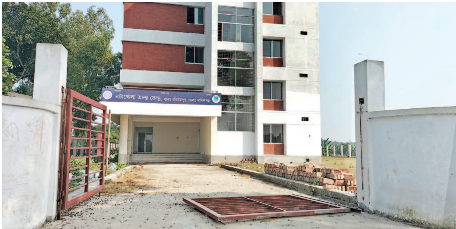
The under-construction building of Natakhol Police Investigation Centre in Manikganj's Harirampur upazila.
