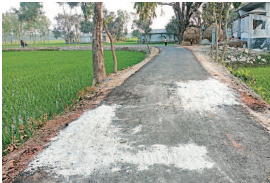
Carpeting of this newly renovated road in Lalmonirhat's Aditmari upazila is getting damaged even before completion of the road work. PHOTO: STAR
