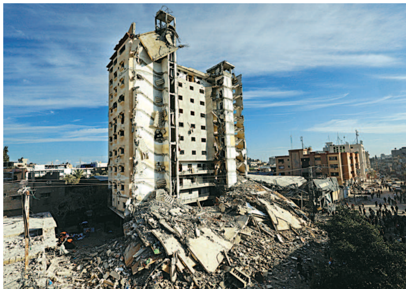
A partially collapsed building after an Israeli air strike in Rafah in the southern Gaza yesterday.
