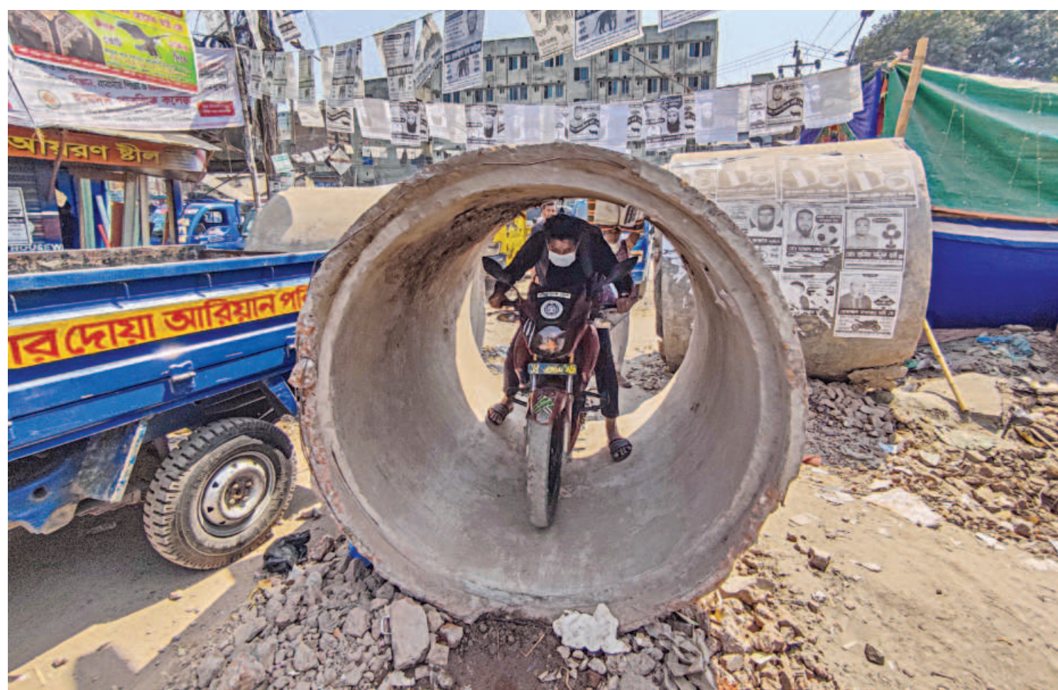
Unable to find an opening to move ahead, a biker tunnels through a sewerage pipe kept on the entrance of Nawab Yusuf Road in the capital's Nayabazar area yesterday noon. The road has been under repair for over two months, obstructing movement of vehicles and pedestrians.
