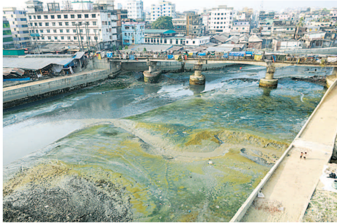
Siltation has almost blocked the Chaktai canal at the place where it merges with the Karnaphuli in Chattogram city. If water does not flow through the canal, waterlogging worsens in parts of the port city in monsoon. The photo was taken yesterday.
