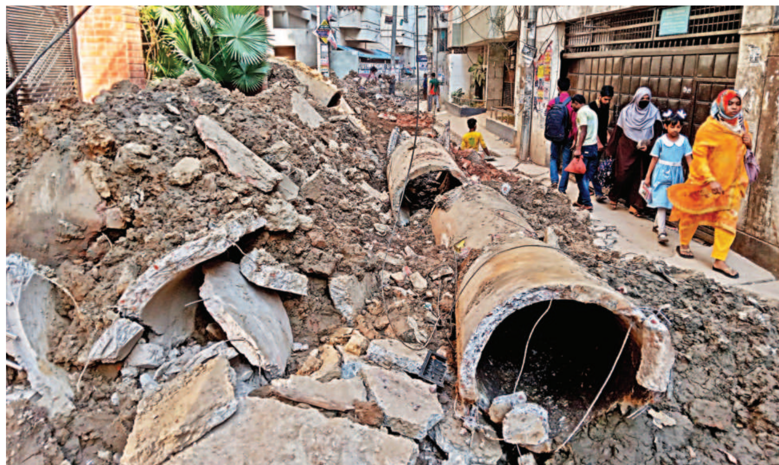
A woman and her school-going child, along with others trailing behind, are having to tread with extreme caution on Moghbazar's Greenway Road, which the DSCC has dug up for development work. The road remains almost entirely blocked for around 15 days now, causing disruptions to people's movement. The photo was taken yesterday.
