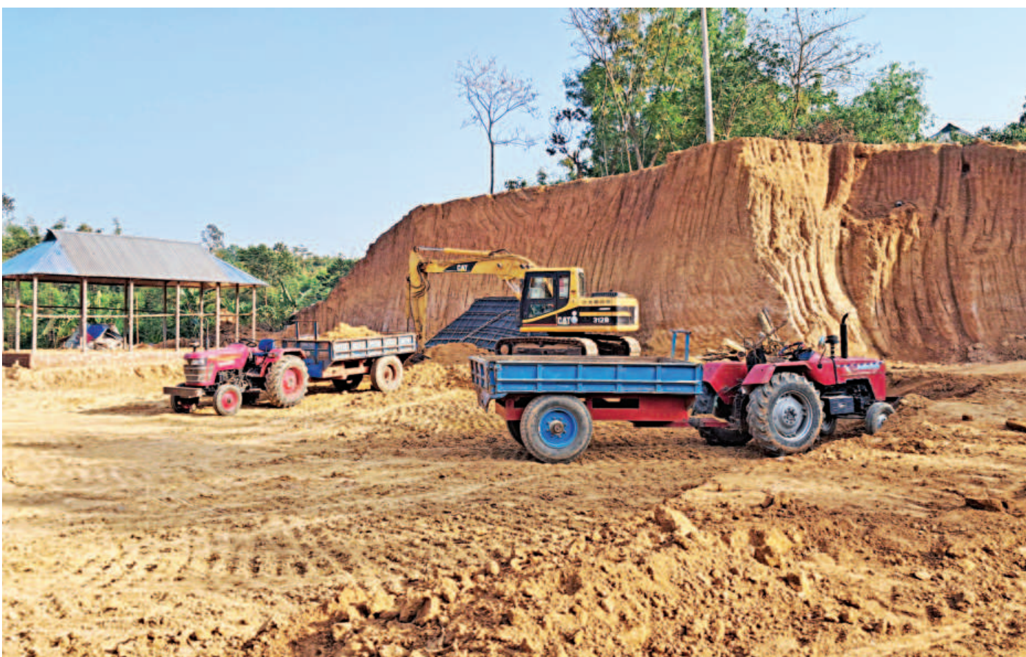
Hills being cut by a syndicate, led allegedly by a local influential, in Brahmanbaria's Kasba upazila. Locals have claimed that the gang has long been cutting hills in broad daylight and selling the soil for illegal gains. According to the Environment Protection Act, no one is allowed to cut hills without permission from the DoE. However, the upazila administration seems to have turned a blind eye towards this practice that is degrading the environment. The photo was taken recently.
