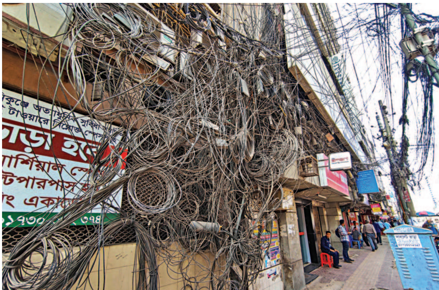
Cables for internet service and satellite TV tangled up in front of a building in the capital's Motijheel area, a common sight across the city. Such haphazardly placed cables are not only an eyesore, they become obstacles for emergency workers in the event of a fire at a nearby building. The photo was taken recently.
