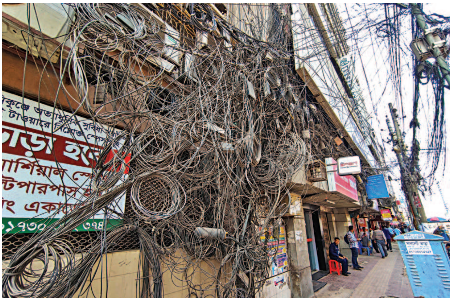
Exposed electric wires all tangled up in front of a building in the capital's Motijheel area, while overhead cables hang chaotically twisted above -- a common sight across the city. Such haphazardly placed electric wires and cables increases the risk of fire incidents. The photo was taken recently.
