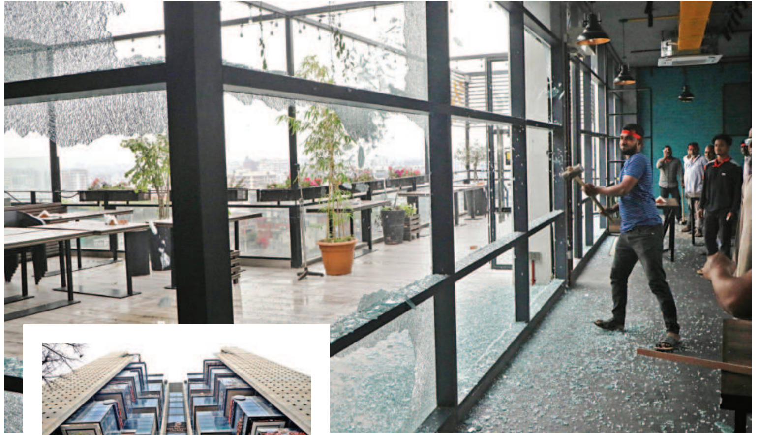
The rooftop restaurant in the Gausia Twin Peak tower, on the capital's Satmasjid Road, being demolished during a drive by Rajuk authorities yesterday. The drive was conducted as the building was constructed for offices and not for housing restaurants. Inset, at least 12 restaurants in the building were sealed off during the drive.
