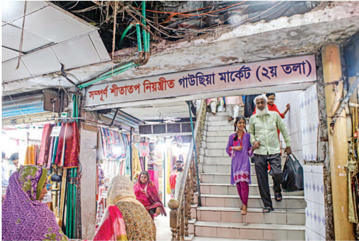
An elderly man leads his family down a narrow stairs of Gausia Market yesterday. The sprawling, congested market lacks the necessary safety measures to safeguard lives if a disaster occurs like the fire in a building on Bailey Road.
