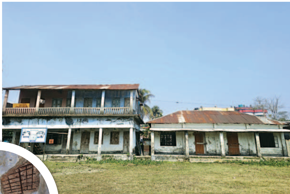
The academic buildings of Amtali MU Girls Pilot Secondary School, the lone educational institution for girls in Barguna's Amtali upazila, lies in a dilapidated state due to lack of repairs and maintenance. All 420 of its students have no choice but to attend classes amid risks.
