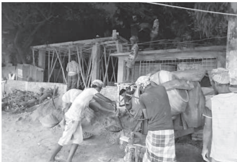
Despite protests, work to construct a public toilet allegedly encroaching upon the land of a Buddhist temple continues. PHOTO: STAR
