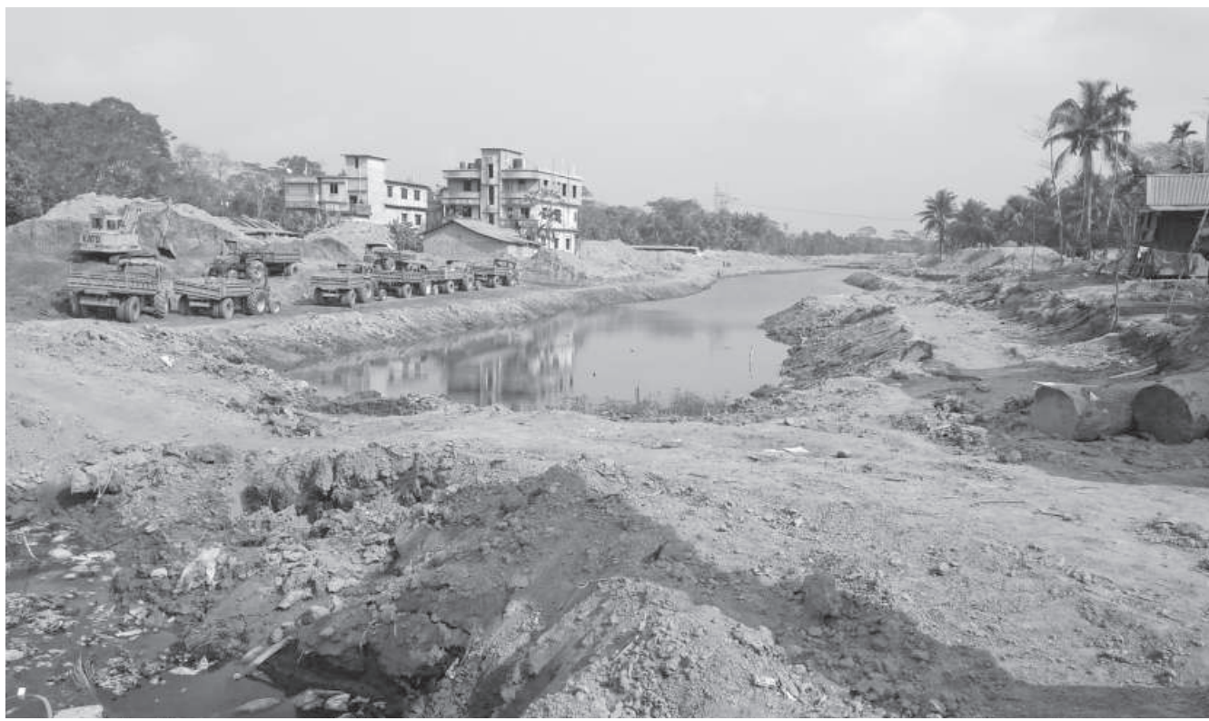
BWDB recently dredged a 23-kilometre stretch of Bishkhali river in Bagerhat, aiming to improve irrigation in the area. However, it is doing exactly the opposite as many acres of croplands, canals and irrigation channels have been dried up as a result.
