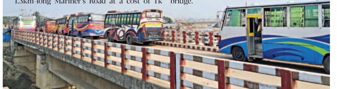
Due to a lack of approach roads, the two-lane bridge over Rajakhali canal in port city's Kotwali area is now being used for parking buses. PHOTO: STAR
