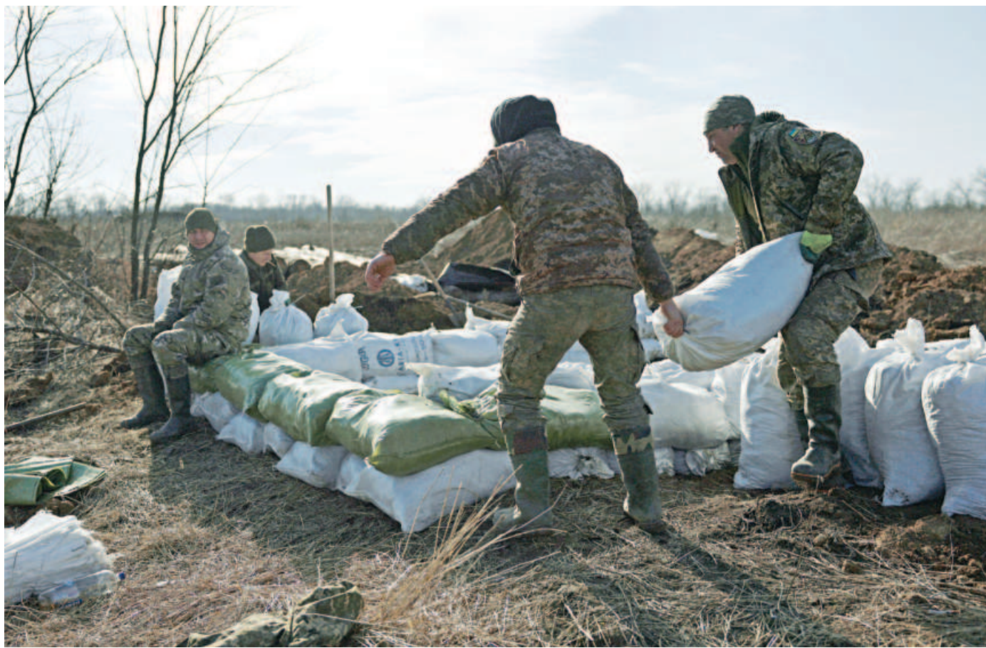
Ukrainian servicemen pile up earthbags to build a fortification not far from town of Avdiivka in the Donetsk region, amid the Russian invasion of Ukraine.
