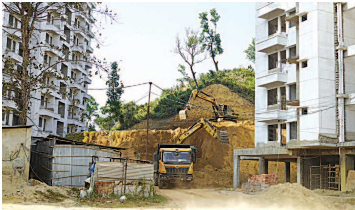
The Cox's Bazar Development Authority has allegedly been cutting some hills inside its high-rise residential apartment project in Kolatoli area of Cox's Bazar town and dumping the earth at a low land in front of the project area. The photo was taken yesterday.
