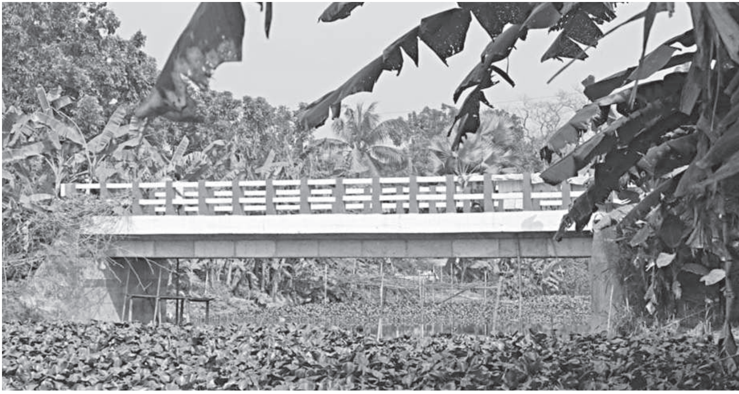
A 15-metre long bridge constructed on the Ichhamati river by narrowing down the waterbody from both ends. Four other such unplanned structures have been built on the river, destroying its natural flow and navigability.
