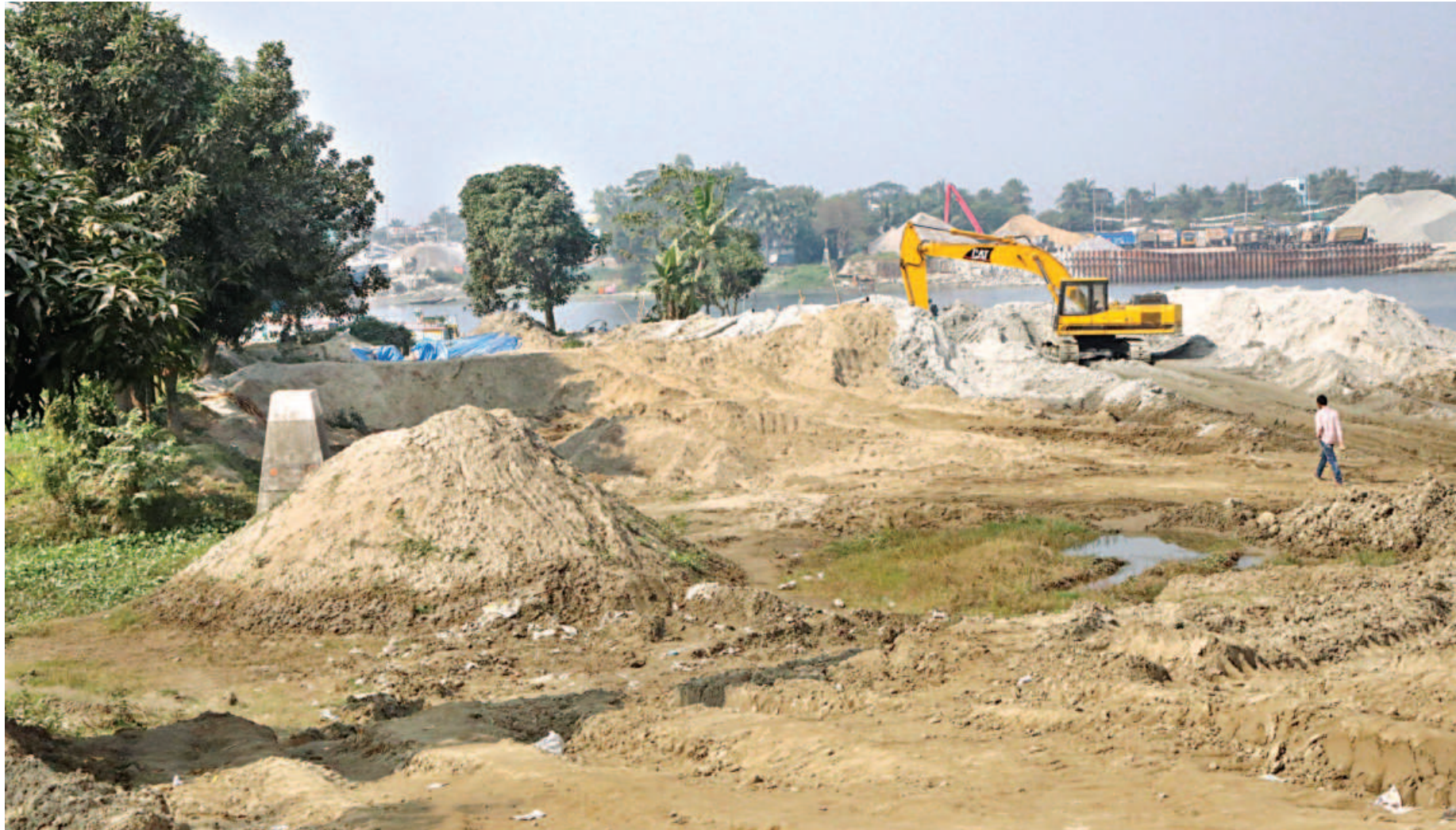
A section of the Shitalakkhya river is being filled at Darikandi of Narayanganj's Rugganj. The pillar on the left of the photo, just behind the pile of dirt, marks the territory of the river. Locals say that the river has significantly shrunk there as traders of sand and other building materials have occupied a large chunk across the river. PHOTO: PRABIR DAS
