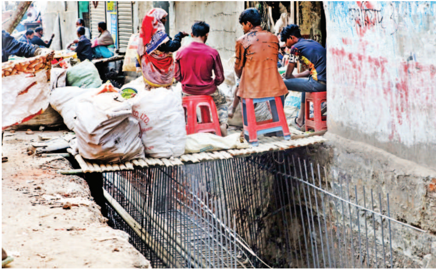
With sacks of scrap materials beside them, shopkeepers sit on stools on a makeshift bamboo platform set up over pointed iron rod extensions of an under-construction road in Kotwali area of Wise Ghat yesterday. Due to the ongoing work, many traders in the area have set up such platforms to walk. However, they continue to use those for keeping sacks and sitting purposes. The structures may collapse as they are not strong enough to endure such heavy weight for prolonged hours.
