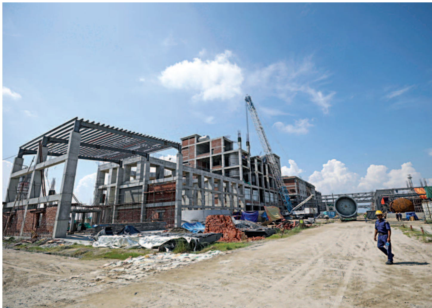
The water demand in the Bangabandhu Sheikh Mujib Shilpa Nagar is projected at 103 crore litres per day, according to sources at Bangladesh Economic Zones Authority.
