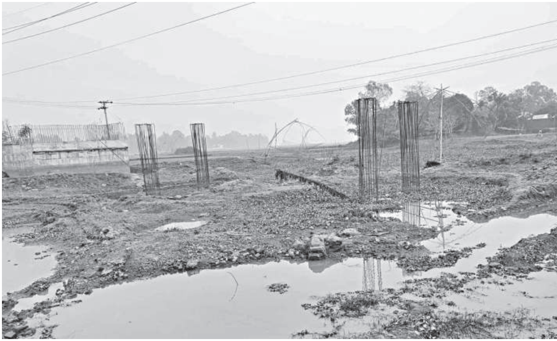
The Khakuriya bridge was supposed to be completed about 2 years ago under a Tk 4.21 crore project. However, the structure remains incomplete, hindering communication across 40 villages in Tangail's Ghatail upazila.
