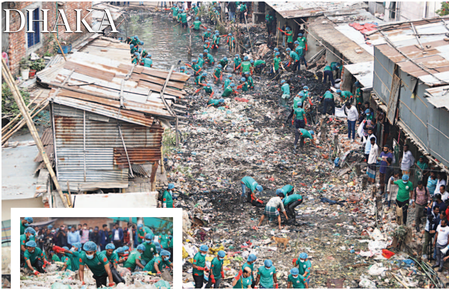
Around 1,200 volunteers of BD Clean along with DNCC began cleaning Mirpur's Paris Canal yesterday. The initiative hopes to restore this canal to its former glory, removing all illegal structures and wastes that have left the waterbody on the brink of death.
